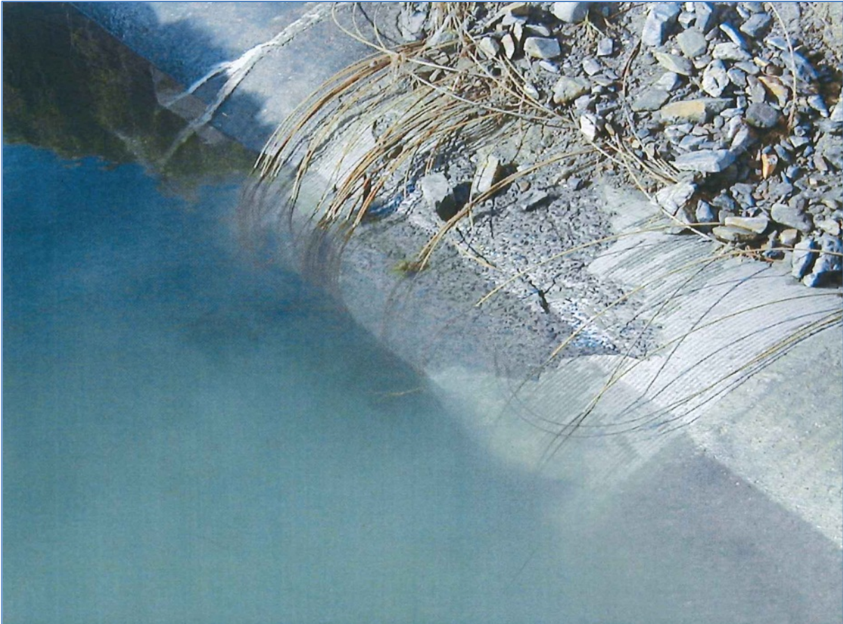
Figure 45: Typical Pipe Burst on the CCT's Potable Water Pipeline from the Voëlvlei Dam
