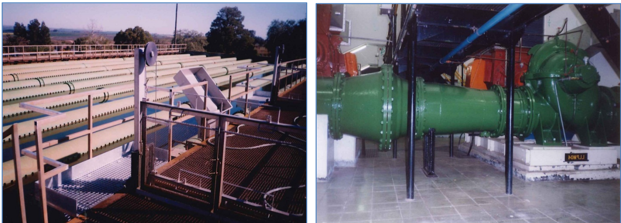
Figure 6: The CCT's Water Treatment Works and Low Lift Pumps at Voëlvlei Dam
